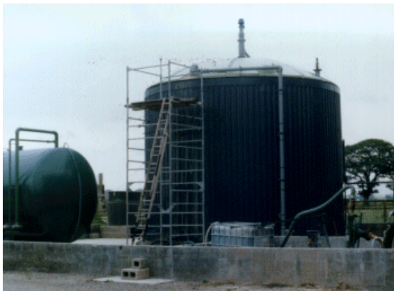
Anaerobic Digester-Farm Size
